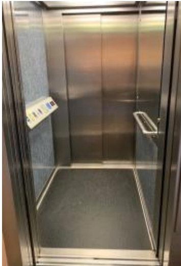
Image shows inside the lift
